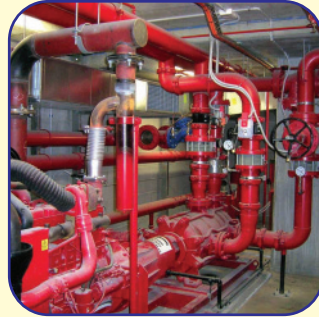
FIRE HYDRANT SYSTEMS
